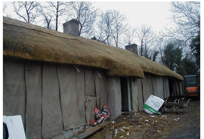
Fig.11 Front and back elevations were draped with hessian covers to speed up the drying process of the external lime mortar and to protect the same from frost while it was allowed to cure. (Photo courtesy of Eddie O'Neill)
