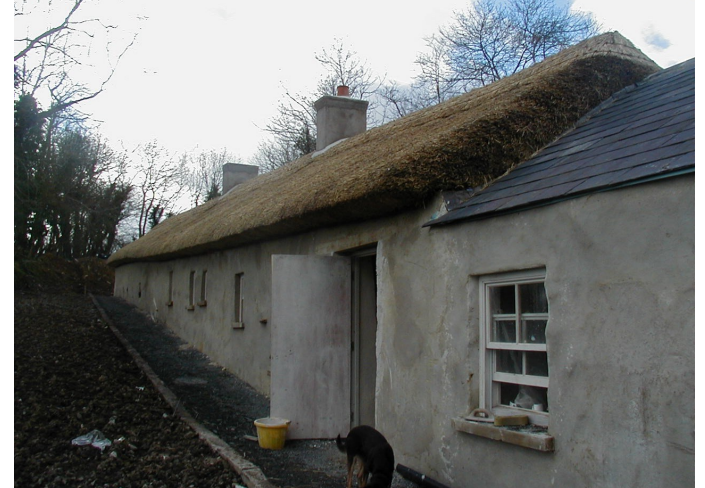
Fig.12 & 13 showing the removal of the hessian covers from the front and back elevations after six months of drying (Photos courtesy of Eddie O'Neill)
