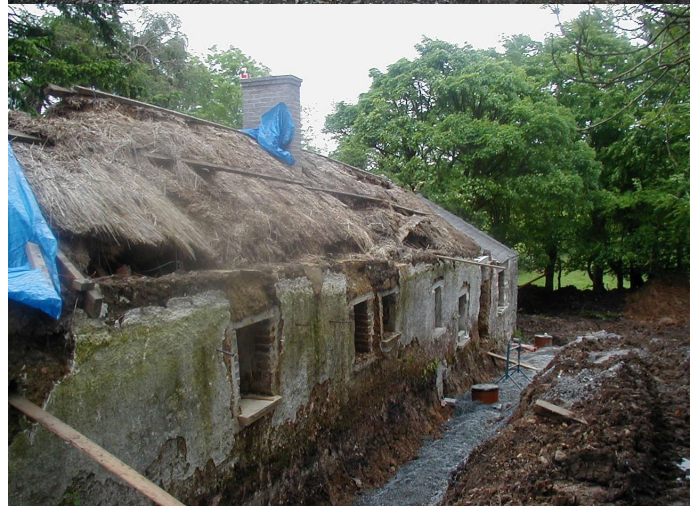
Fig.4 & 5 showing front and back elevations with damaged materials removed. This was based on respect for the existing fabric i.e. minimum intervention. The least loss of the original fabric i.e. maximum retention (Photos courtesy of Eddie O'Neill)
